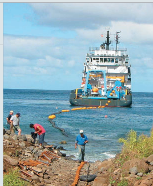
Deployment of near shore cable at hydroacoustic station HA3, Juan Fernández Island, Chile. The floats holding the cable at the sea surface are later removed, allowing the cable to sink to the sea floor.
