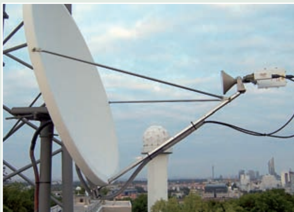
New radio frequency transmitter-receiver head installed on the antenna of the Austrian National Data Centre, Vienna.
