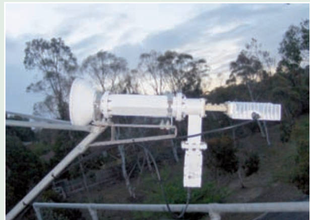
New radio frequency transmitter-receiver head installed at a GCI VSAT site providing communications for radionuclide station RN4 and radionuclide laboratory RL2 in Melbourne, Australia.
