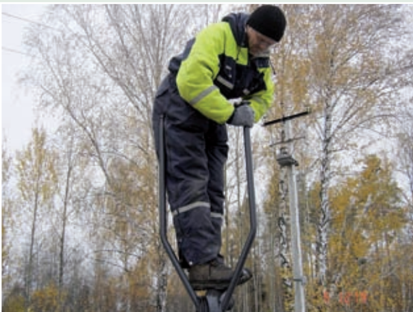
Installation of a Global Positioning System unit at primary seismic station PS33, Zalesovo, Russian Federation.
